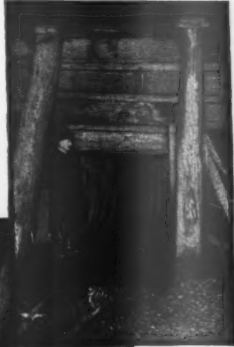
ON THE UPPER SIDE OF THE FLOOD GATE, WHERE TIMBERS THICKER THAN A MAN'S BODY SUPPORT THE WALL.
